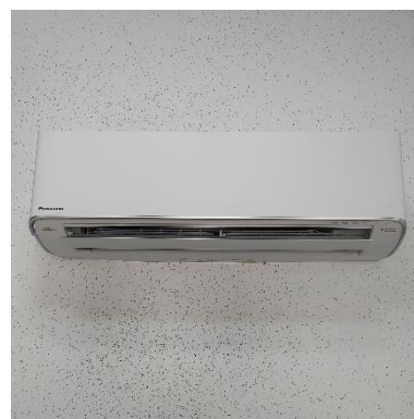
Panasonic Air condition
